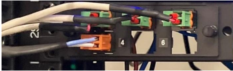
Connector Assembly in Patch Panel
